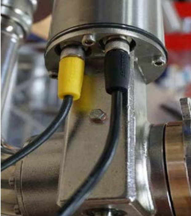
Phases and Sensor cable to vertical motor
